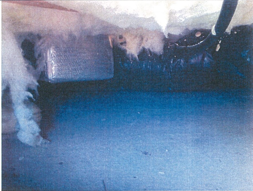
116 Demmy Avenue, Ducting in Crawlspace, 04/14/13
